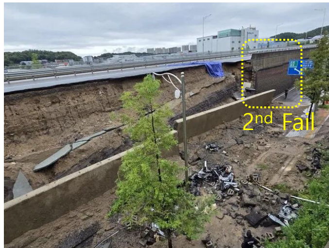
1 st Failure (July 2025)
